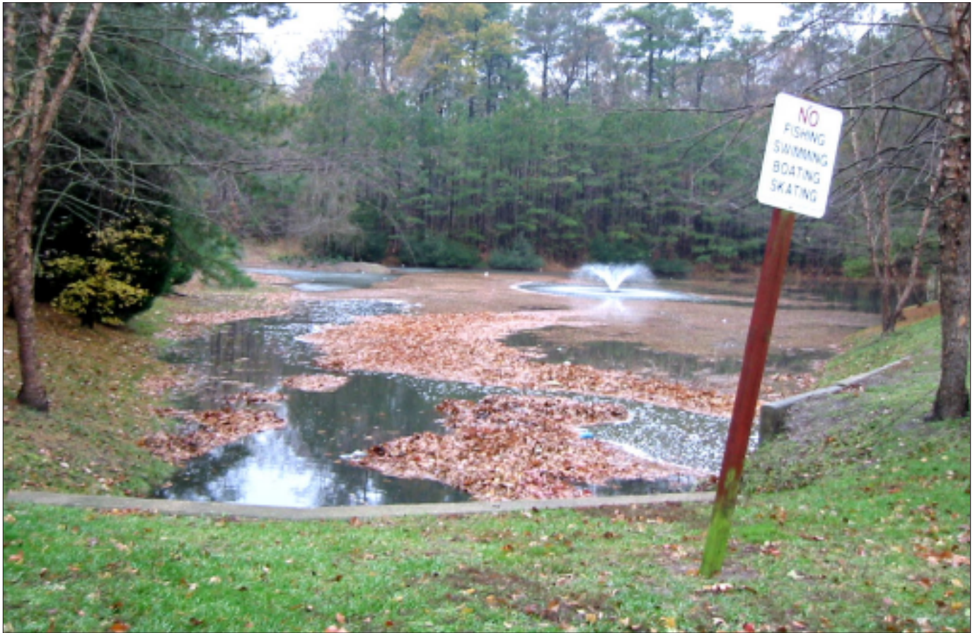
UNTIMELY DEMISE: Of the ponds that fail in the first five years, over half of them fail due to lack of proper maintenance.
