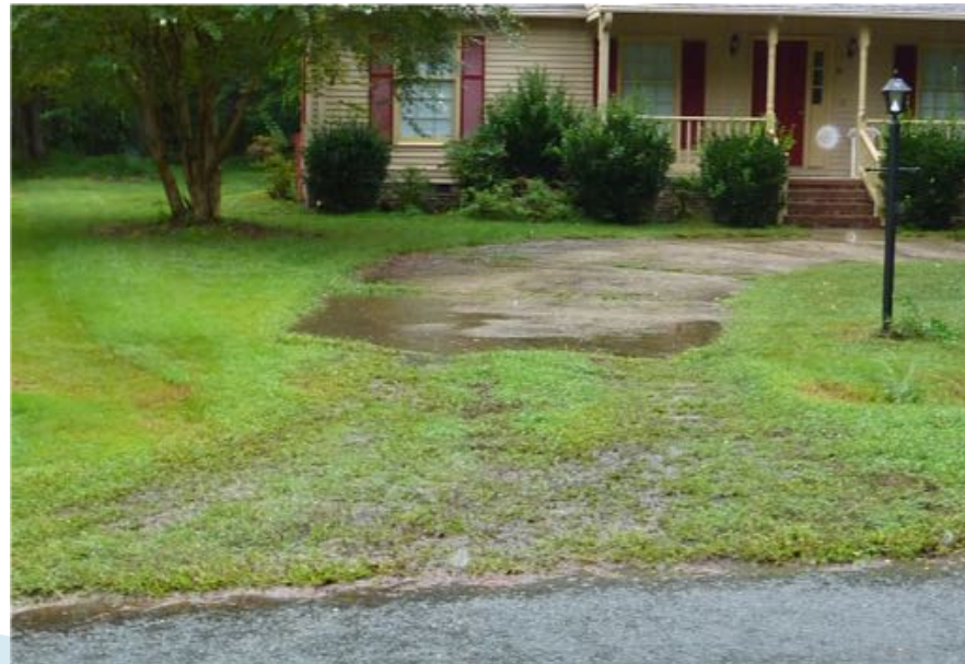
Overgrown Driveway Apron
